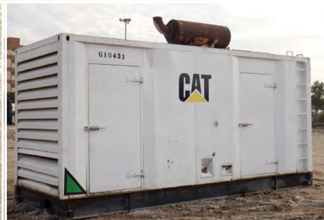
2013 CAT 550 500 KVA CONTAINERIZED
